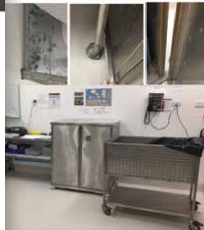
it is the replacement of items that have significant rust damage control risk which was mostly noted in the Wash Area. Items raspase as required.
